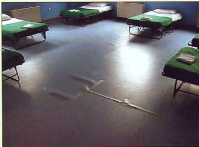
Excessive moisture and high pH in concrete floors can cause many modes of floor covering failures. A typical type of distress is debonding of adhered floor coverings, which form large bubbles and tripping hazards at joints.
